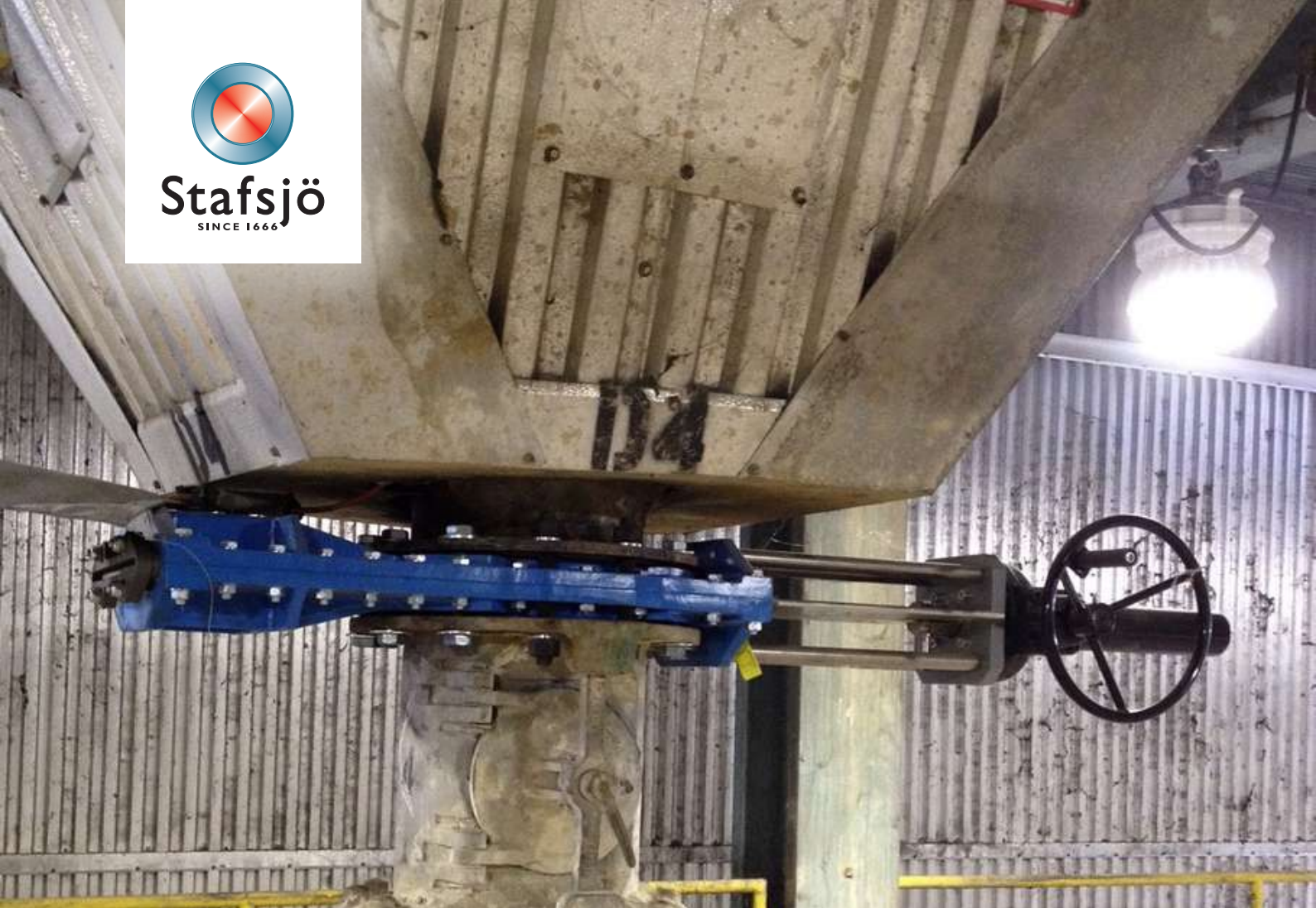
The HG-L installed on a ash hopper
